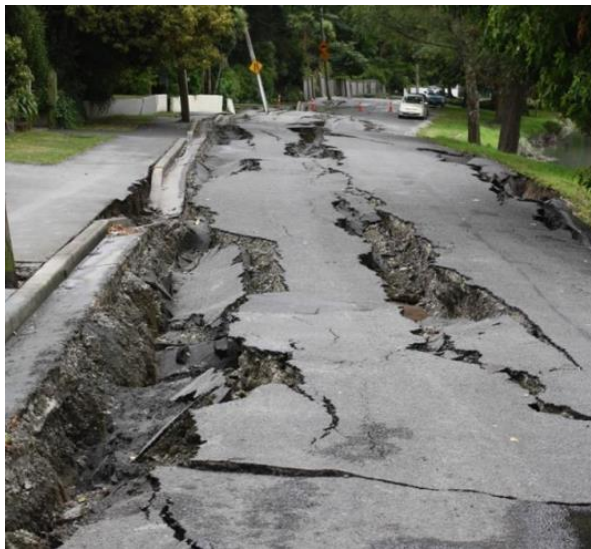
Figure 2.7 - Effect of lateral spreading on the roadway after the 2011 earthquake series in Christchurch (New Zealand).
