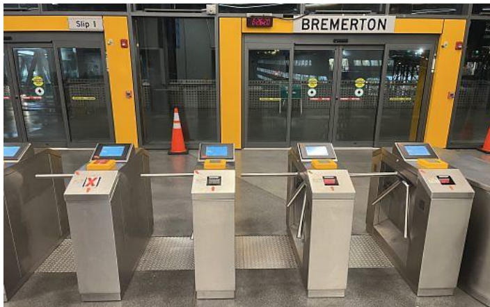
Figure 5.17 Entry to a terminal showing automated turnstiles and access indicators
