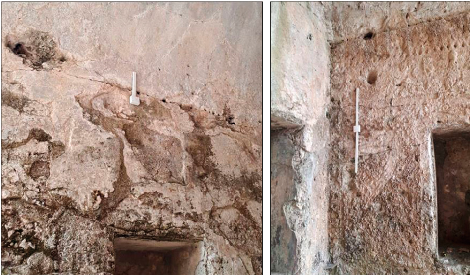
Fig. 5 – Two of the FBGs installed at two major cracks.
