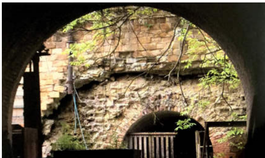
Fig. 2 - Roma, Forte Antenne, Dissesti nelle murature perimetrali. (Source: created by the authors)
