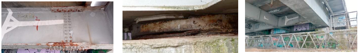
Fig. 5. (a) corrosion of the connections, (b) shrivelled part of bearing, (c) inspection bench and the view on the longitudinal and transversal beam of bridge deck.
