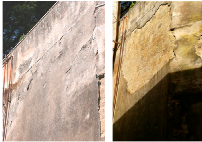
Figure 10. Retaining wall built in Neapolitan Yellow Tuff dimension stones in 1957, coated by a layer of plaster (Parco Grifeo, center of Naples). The picture on the left portrays the wall as it appeared in 2011, whereas the picture on the right portrays the same wall as it appeared in 2014 after the separation of the plaster (picture by M. de Gennaro).
