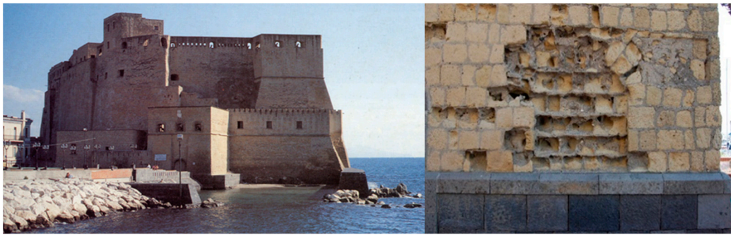
Figure 11. Example of the marked physical weathering of facia vista Neapolitan Yellow Tuff dimension stones, consisting of a marked consumption of their exposed surface assuming a typical concave shape (Castel dell' Ovo, center of Naples, left: whole building, right: physical weathering; picture by A. Langella).
