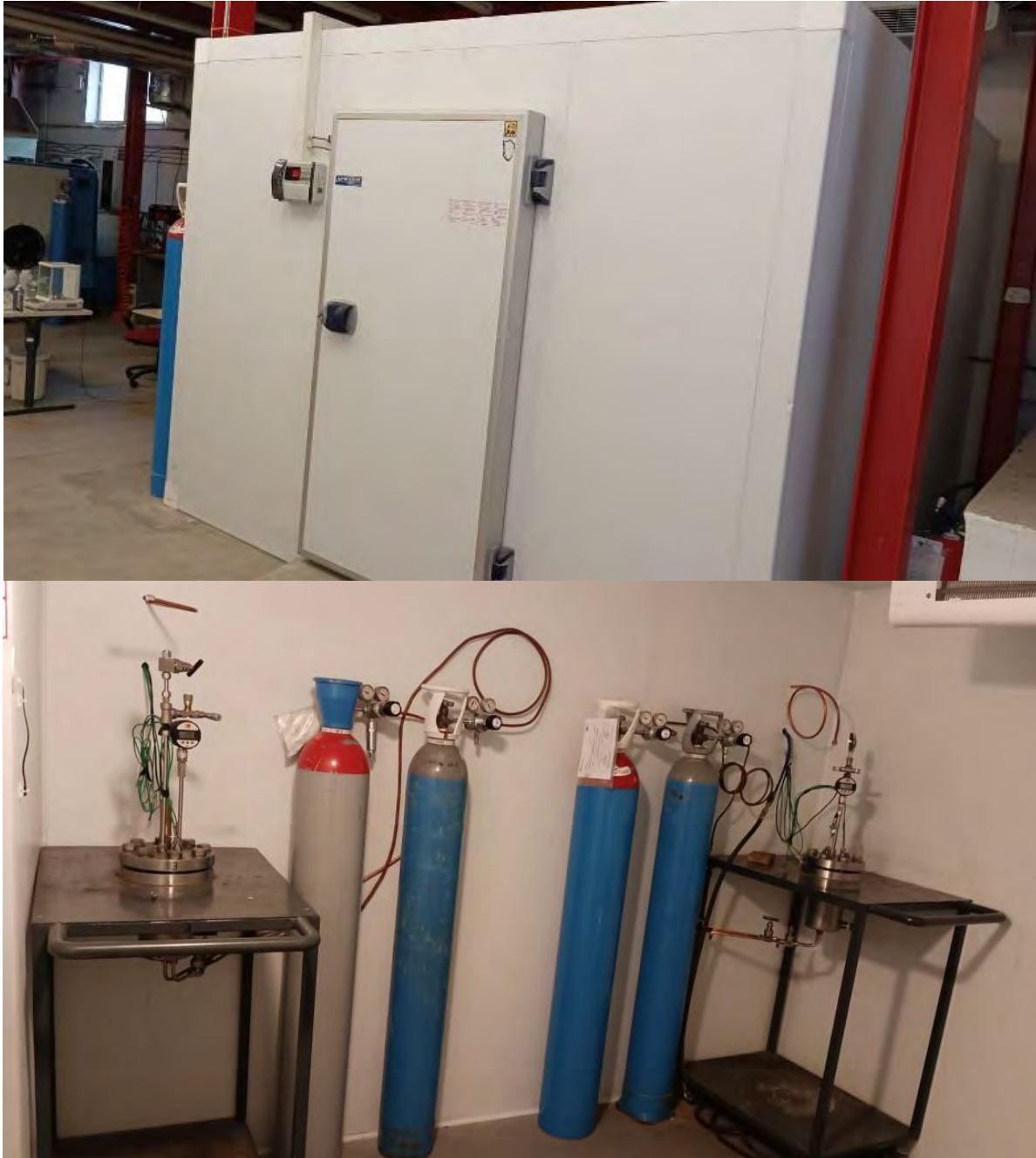
Figure 5. The new reactors in the refrigerated room.
